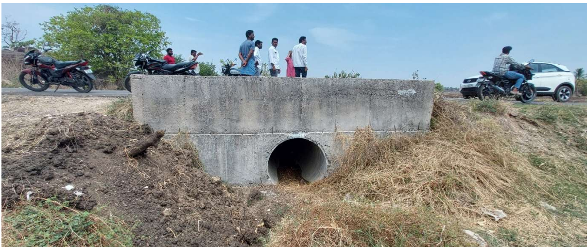
Pic 13, 14 & 15 – View of the pipe culverts supporting effective stormwater drainage.
